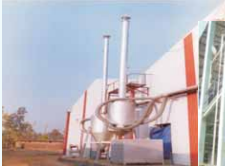
Wet Scrubbers and Cyclones
