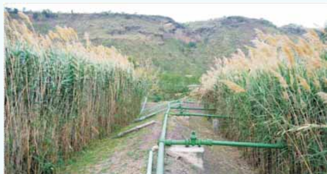
Root Zone Biotech plant at ACC Gagal
