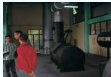
Incinerator at MC Shimla
