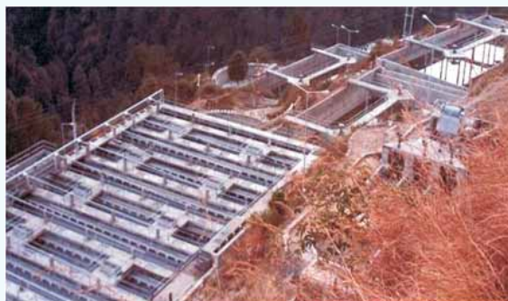
Treatment System for Treatment of Domestic Waste Water (Source-SPCB)
